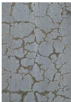
Typical surface crack pattern for ASR
