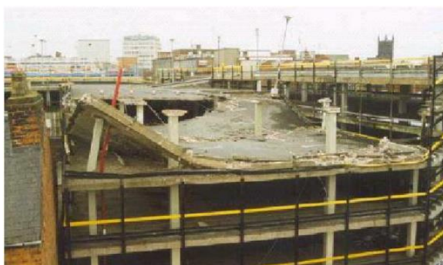
Pipers Row car park after the collapse
