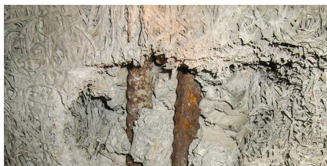
Exposed reinforcement with woodwool formwork
